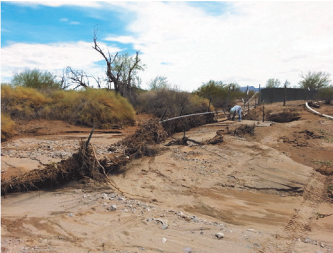
Storm Damage, July 2014
