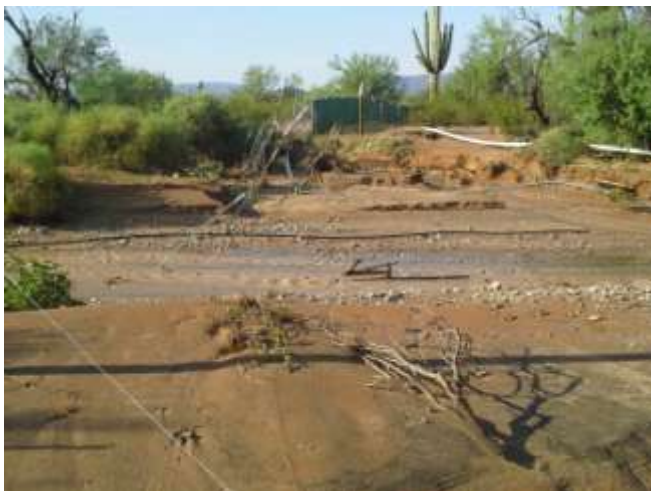
Storm Damage, August 2014
